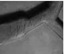
Cracking Between Tread
